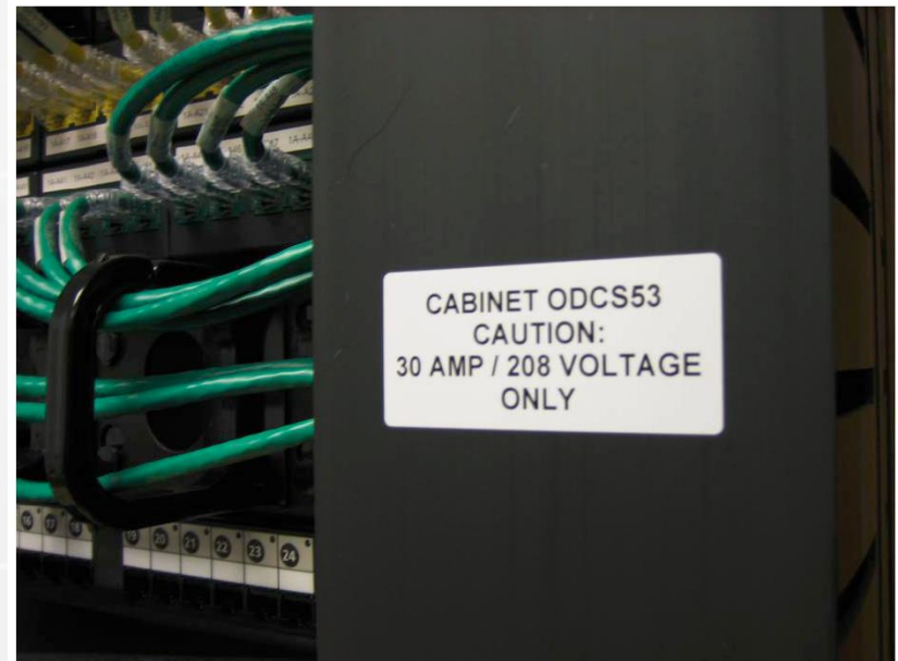
IBM Application – Rack Labels
