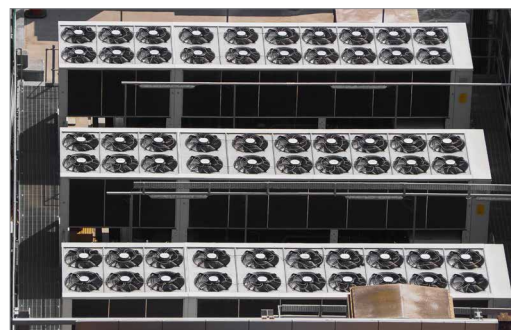
Heating, ventilation and air conditioning unit
