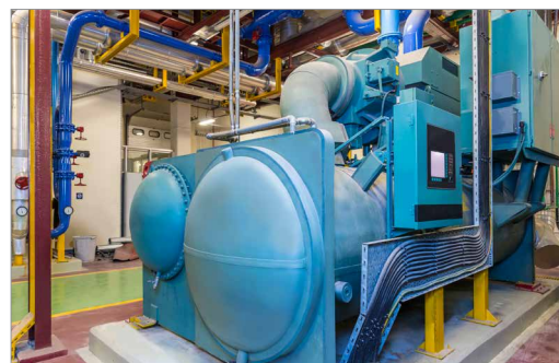
Chiller for active cooling
